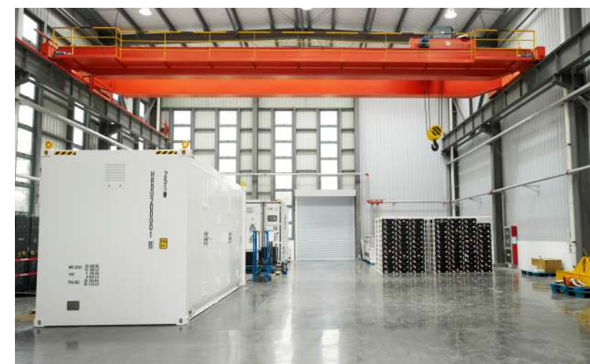
Containerized Utility Battery Workshop
