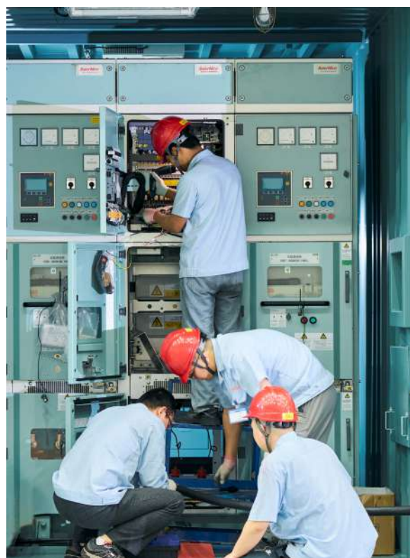
HV Switchboard Workshop
